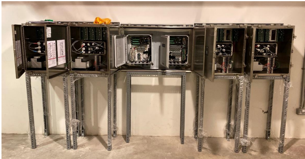
Figure 4. Data loggers of the Al-Hamra Tower's Structural Health Monitoring system.
