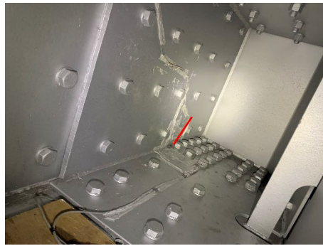
Figure 4. Torsion box retrofit located inside the gate. The location crack through the plate behind the retrofit is indicated with a red line.
