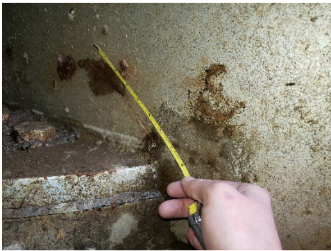
(a) Skin plate crack
