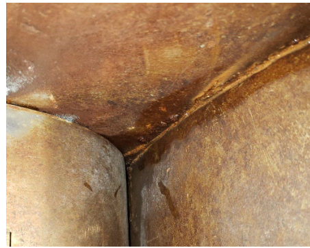
(b) Girder web crack
