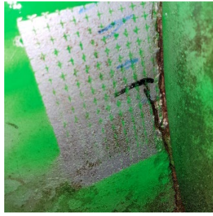
Figure 3. Web crack with grid
