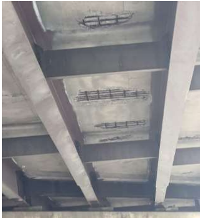
Figure 2 Highway overpass bridge with multiple delaminations of concrete on underside of the deck
